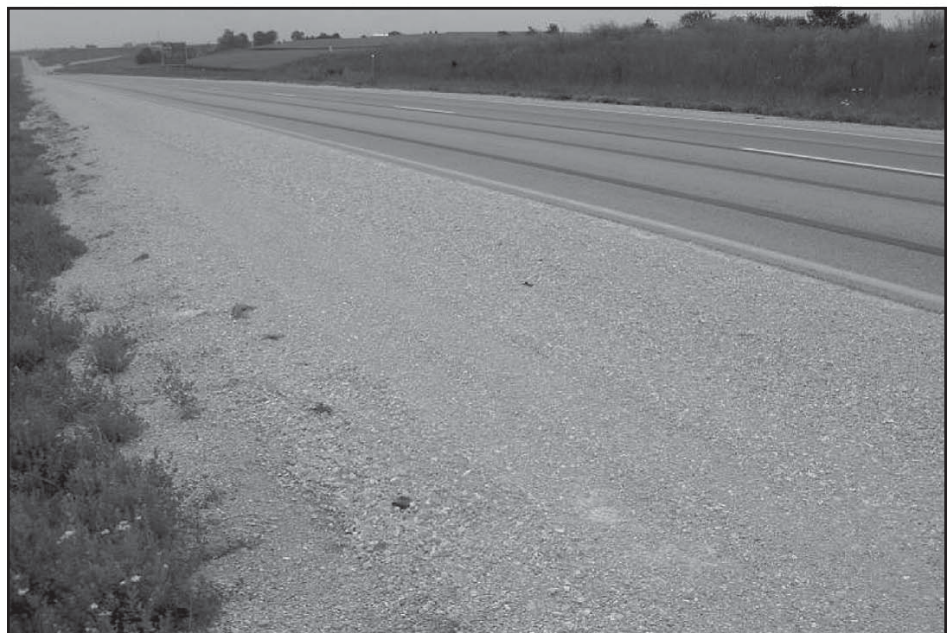
Figure 2. Rutted, unstabilized shoulder (top) Another shoulder area seven months after being stabilized with fly ash (bottom)
